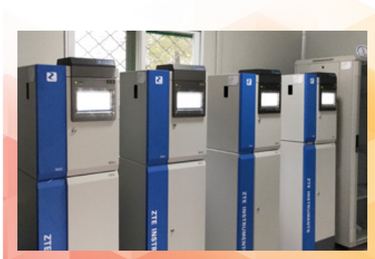
南昌工廠廢水在線監測系統 Wastewater online monitoring system in Nanchang factory
