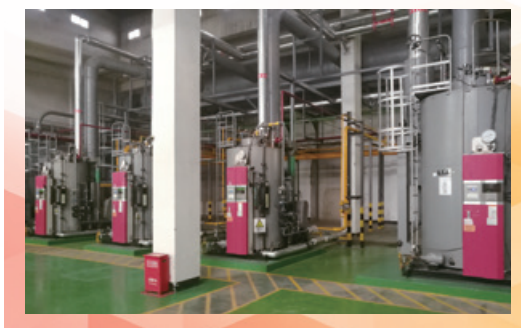
長春工廠天然氣鍋爐 Natural gas boilers in Changchun factory
